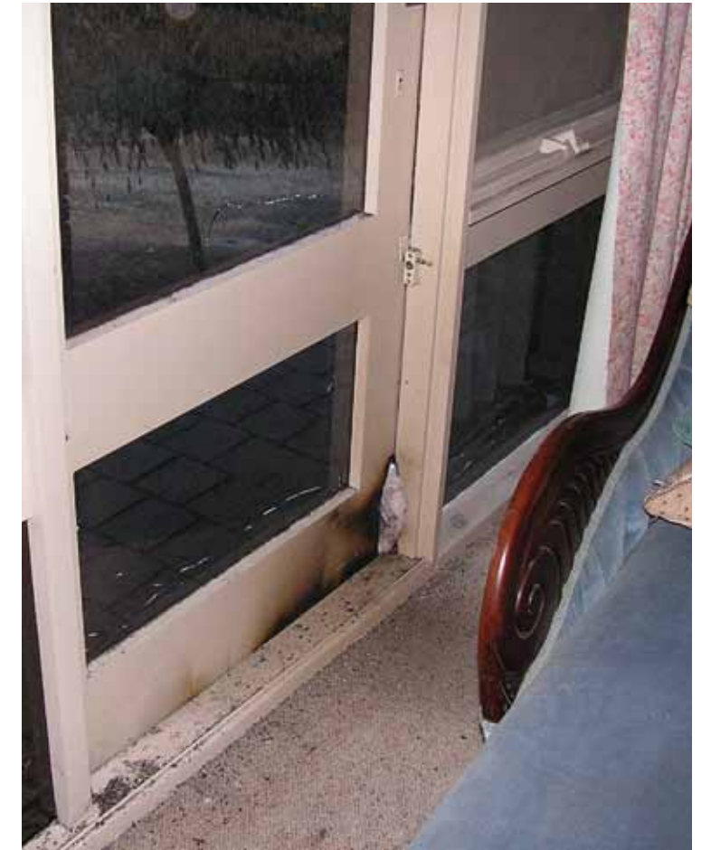
Above: Flames crept under the door damaging the interior of the house.
